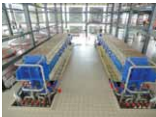
Dry Fractionation Plant - Membrane Press Filter for Separating Liquid Oil (RBD Olein) and Solid Oil (RBD Stearin)
