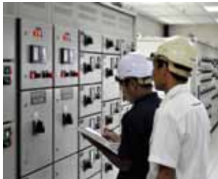
Recording Of Plant Parameters & Utilities Consumption At Refinery
